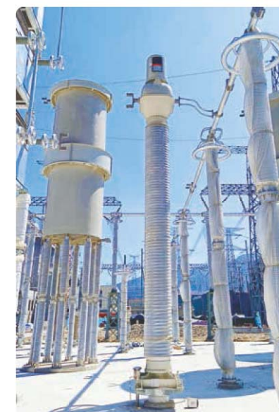
Baihetan - Zhejiang \pm 800 kV ultra-high voltage DC transmission project
