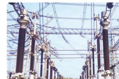
Qinghai - Henan \pm 800 kV ultra-high voltage DC transmission project
