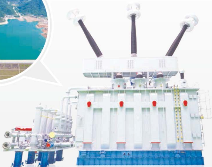
SSP-480000/500 pumped storage transformer is used in Yangjiang pumped storage power station in Guangdong Province
