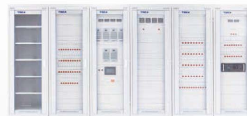
AC and DC Power Systems
