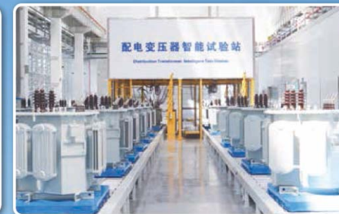
Distribution Transformer Intelligent Test Station
