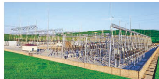
Datka 500kV Substation in Kyrgyzstan
