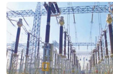
Baihetan - Jiangsu \pm 800 kV ultra-high voltage DC transmission project
