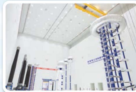
Ultra-High Voltage Bushing Testing Hall
