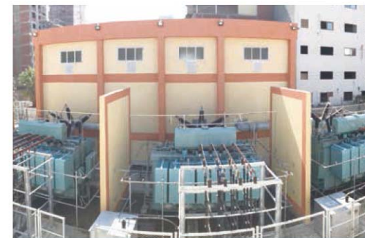
Egypt DAMIETTA EAST 66kV GIS substation
